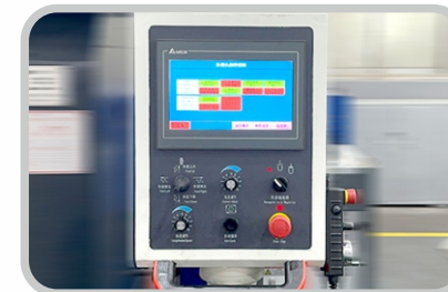
Omron PLC with touch screen
