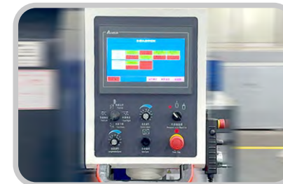
Omron PLC with touch screen
